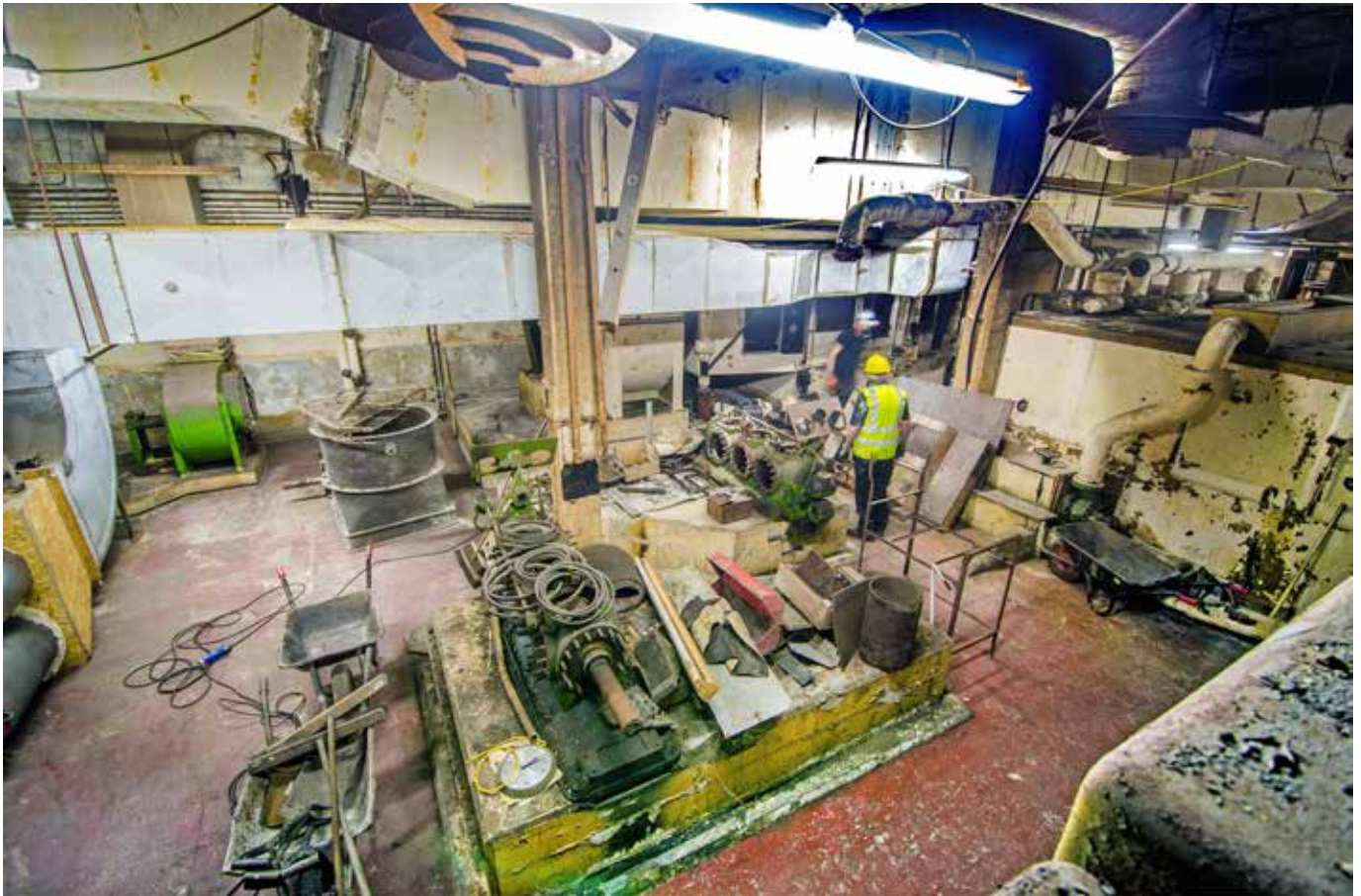
Looking down into the R4 plant room. This is during our clear-out. Bottom left you can see the temporary recirculation fans that we've fitted to provide air circulation while we work. We'll be restoring the main air fan (centre) as part of the project
